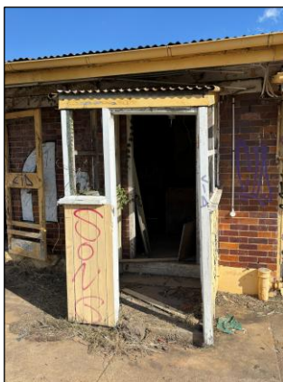
Image 81. Deteriorating timber entry (Apr 26).
