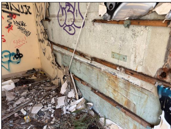
Image 76. Termite damage to wall framing (Apr 26).
