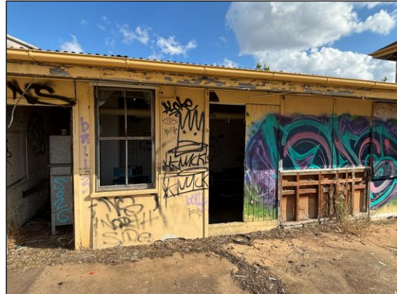
Image 84. Broken asbestos sheet and termites in wall framing (Apr 26).
