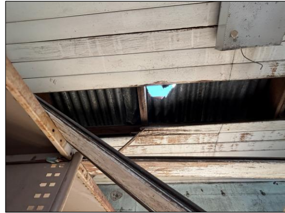
Image 78. Collapsing ceiling (Apr 26).
