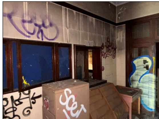
Image 63. East wing entry looking north showing scored render walls (Jan 26).
