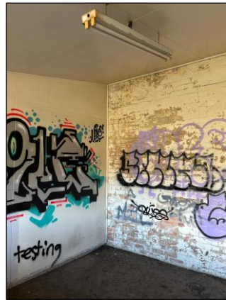
Image 91. Asbestos wall and ceiling sheeting (Apr 26).
