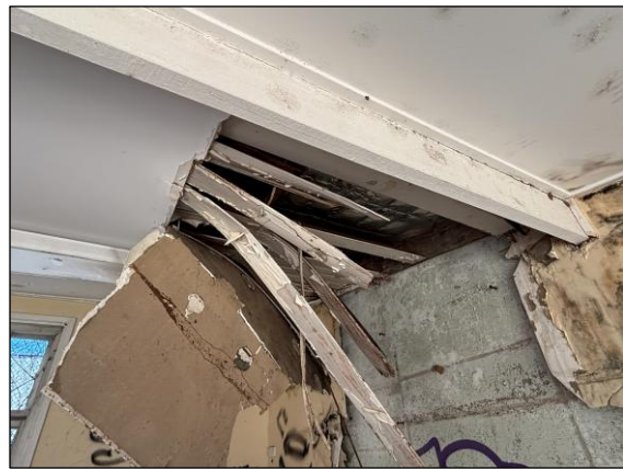
Image 75. Collapsing ceiling (Apr 26).
