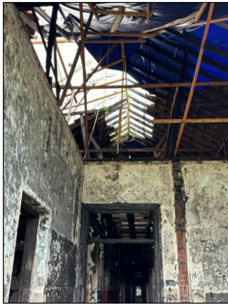
Image 40. South wing fire damage viewed from an external window (Jan 26)
