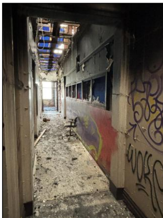
Image 44. East wing central corridor looking south from entry into fire damaged area (Jan 26).
