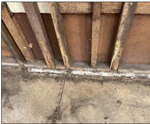
Image 85. Detail of termite damage to north wall (Niche 2024).
