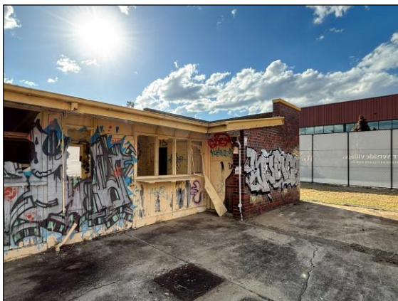
Image 96. Broken FC sheets (Apr 26).
