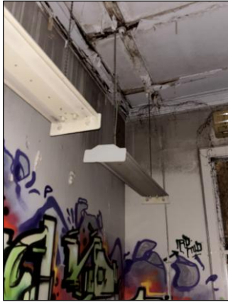
Image 58. North wing south side damaged ceiling from water ingress (Jan 26).
