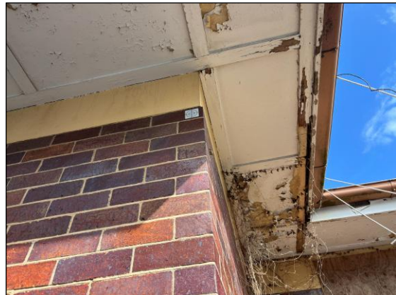
Image 39. Water damage to eaves soffit (Apr 26).
