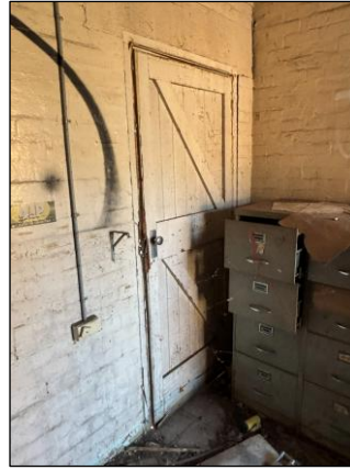
Image 89. Termite damage to door and frame (Apr 26).
