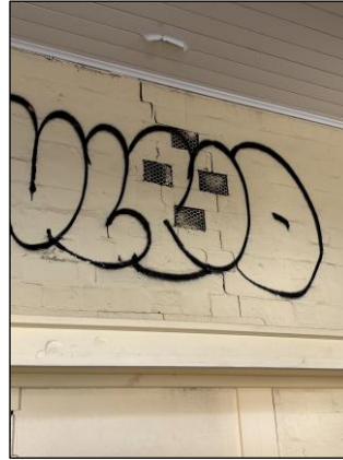
Image 95. Cracks in brickwork (Apr 26).
