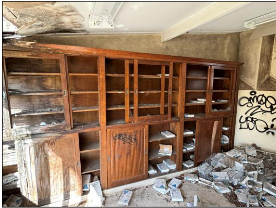
Image 72. Damaged built-in furniture (Apr 26).
