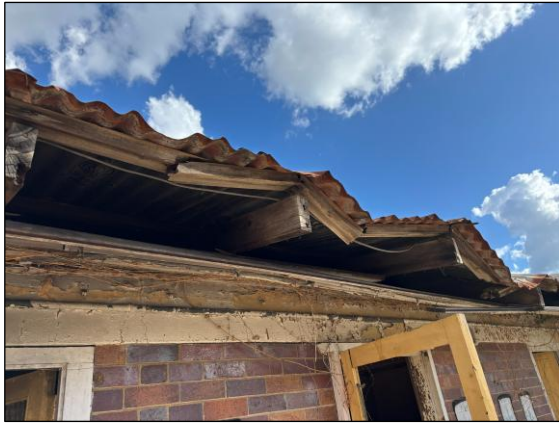
Image 77. Collapsing roof framing (Apr 26).
