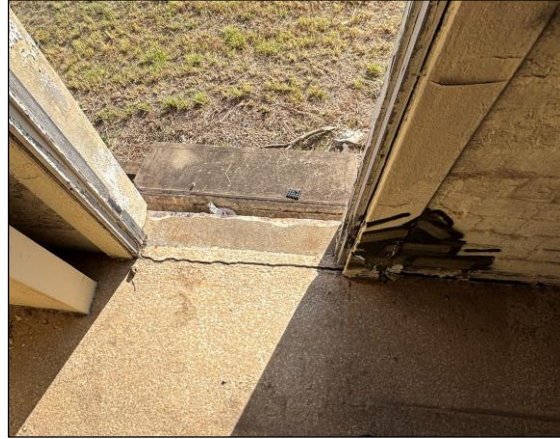
Image 101. Cracks in concrete floor (Apr 26).
