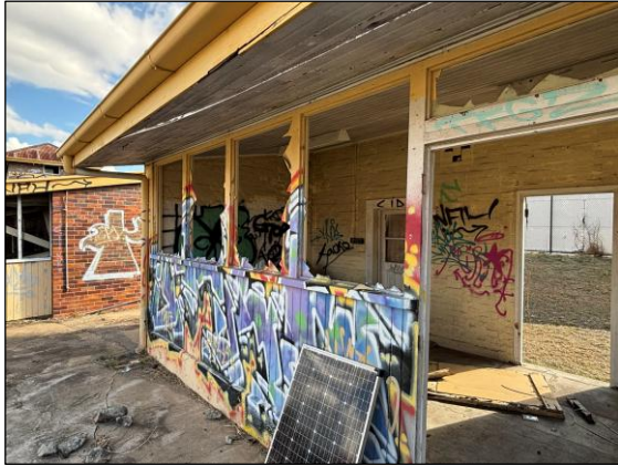
Image 94. Broken glass and removed door (Apr 26).
