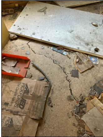
Image 100. Cracks in concrete floor (Apr 26).
