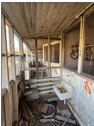
Image 92. Damaged timber to entries (Apr 26).
