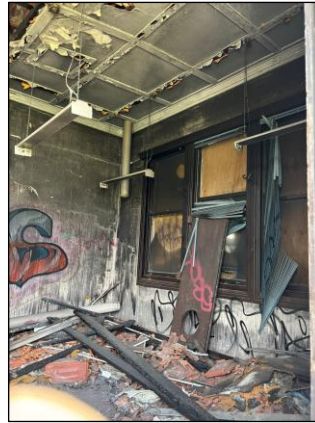
Image 43. South wing fire damage viewed from an external window (Jan 26).
