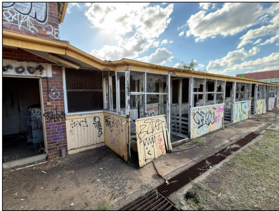
Image 90. Dislodged and rot in timber (Apr 26).
