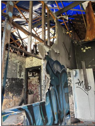
Image 42. South wing fire damage viewed from an external window (Jan 26).
