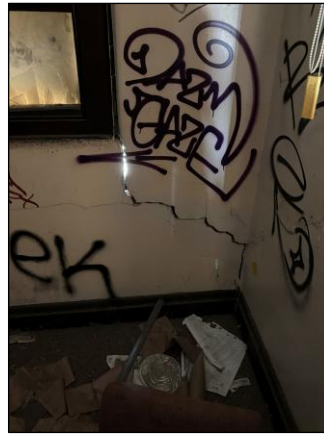
Image 53. North wing meeting room, substantial cracking to external wall (Jan 26).
