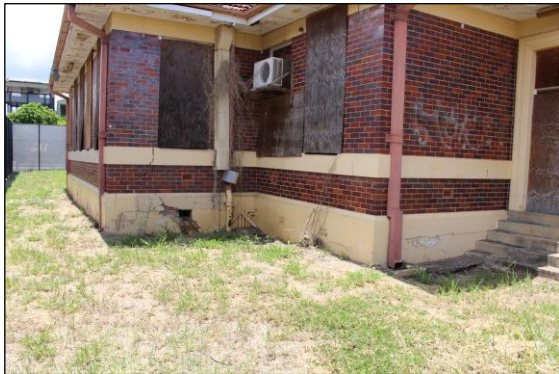
Image 26. North wing part north elevation looking east showing substantial subfloor cracking (Jan 26).
