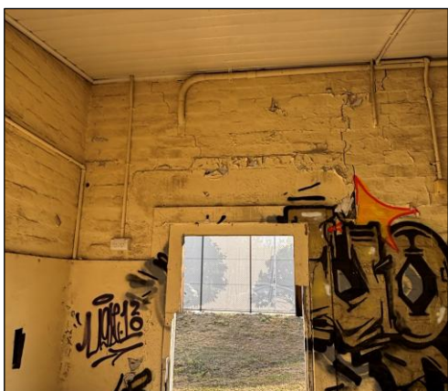
Image 98. Cracks in brickwork above doorway (Apr 26).
