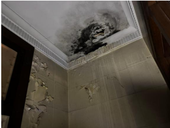
Image 66. East wing entry water damage to plaster ceiling (Apr 26).
