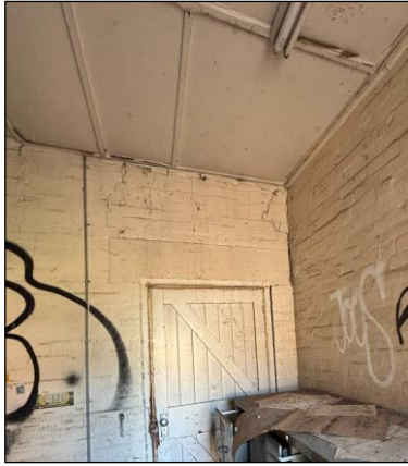
Image 88. Damaged ceiling possibly from water ingress (Apr 26).
