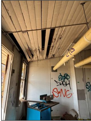
Image 83. Collapsing boarded ceiling (Apr 26).
