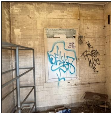
Image 79. Cracks in brickwork (Apr 26).
