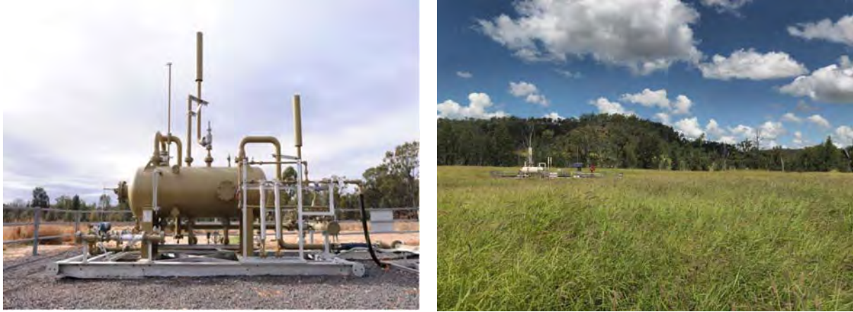
Figure 1-2 Typical CSG wellhead separator and an operating Australia Pacific LNG gas well following rehabilitation of the well lease
