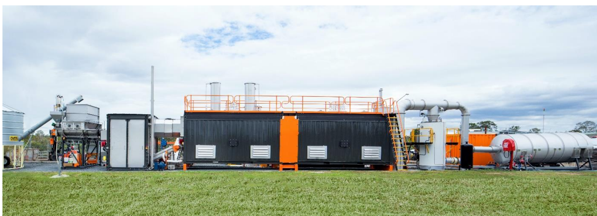
Demonstration plant located at Loganholme wastewater treatment plant, showing full processing system. Image courtesy of Pyrocal.
