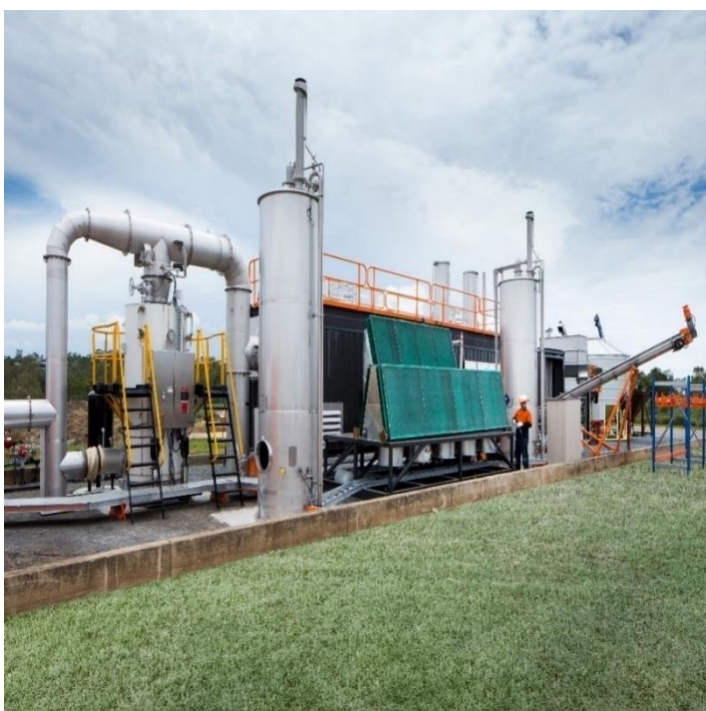
Demonstration plant located at Loganholme wastewater treatment plant, showing heat recovery system. Heat recovery unit and biosolids feed equipment are visible in the background. Image courtesy of Pyrocal.
